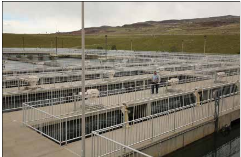
Prioritizing surface water at Jordan Valley Water Conservancy District's 180 mgd plant led to considerable energy savings in phase 1 of the district's energy optimization program. Photo courtesy of JWVCD
